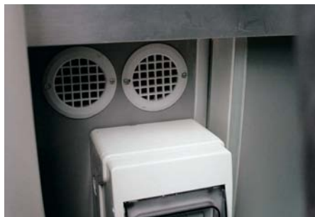
Additional ventilation fitted to front of the unit to improve air flow from the compressor
