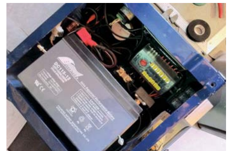
Battery and DC wiring including fuse box, charger shunt and battery monitor all neatly fitted under passenger seat
